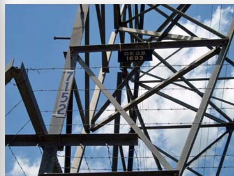
Transend test pylon
