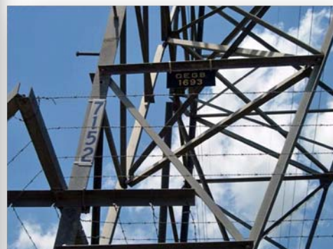
Transend test pylon
